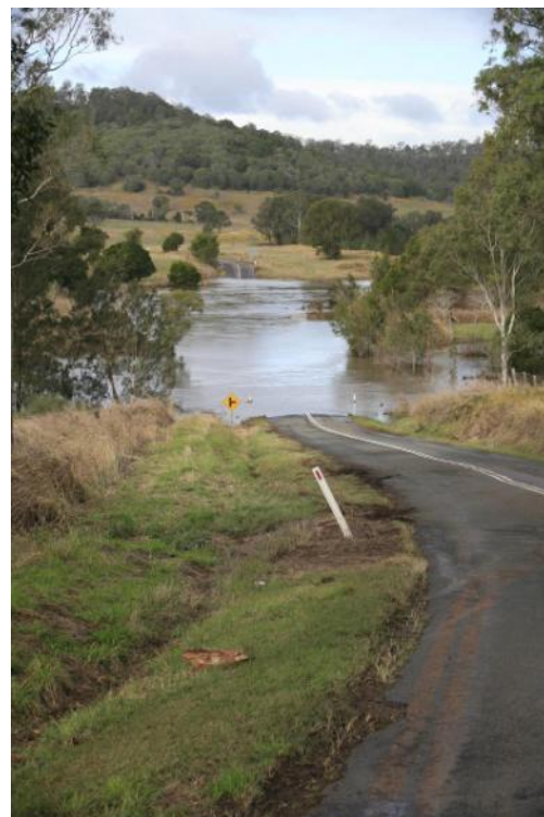
Flood levels at Traveston Crossing Bridge (Photo A. Mackay)
